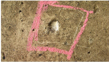
图1 衬砌混凝土表面软骨料的典型表象 Fig. 1 Typical appearance of soft aggregate on lining concrete surface
